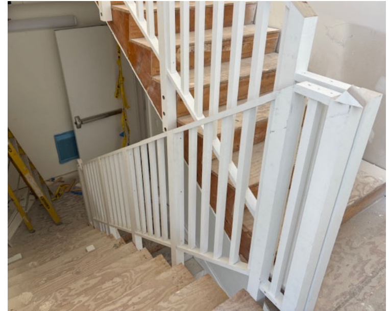
Railings in Egress Stairs Installed
