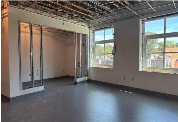
Epoxy Floors in Ceramics Room
