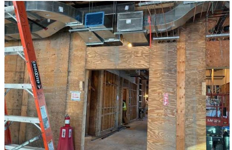
Ductwork and overhead piping
