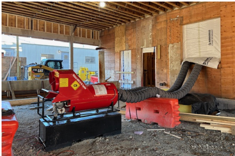
Temporary Heating in Place
